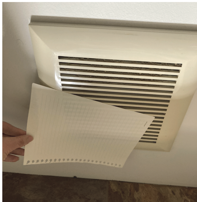
Figure 6 Confirmation of exhaust fan operation using a sheet of paper. Source: Amy Musser
