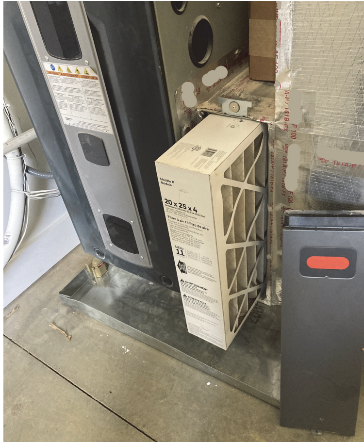
Figure 8 Tightly fitted, high-MERV filter in central air-handling unit. Source: Amy Musser
