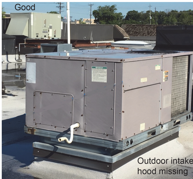
Figure 16 Rooftop HVAC units, including one with a missing ventilation hood.
