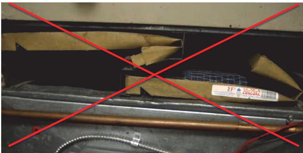
Figure 9 How not to install air filters in an air-handling unit. Source: Schoen Engineering Inc. Reprinted with permission.
