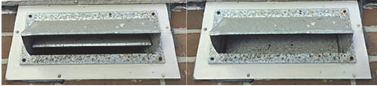
Figure 7 Exhaust fan outlet dampers: open (left) and closed (right).
